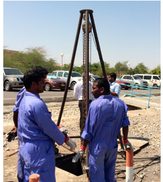
Operators of a pump station located at one of the student residences of the Sultan Qaboos University, install Flygt Concertor.
